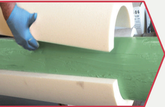
Tank, Line and Process Vessel Corrosion Protection
