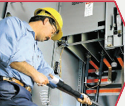
Electrical Construction Materials & Repair
