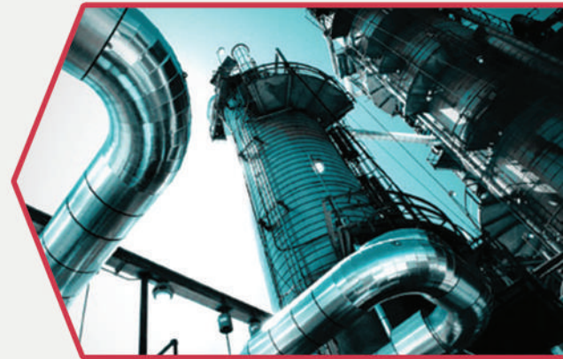
Refinery & Processing Filtration
